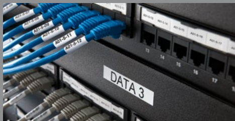
Wire & Cable Identification
