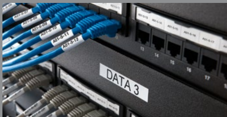
Wire & Cable Identification
